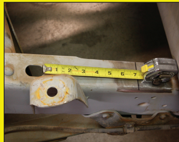
The location of the mount on the rails was established by measuring from a hole in each rail.
