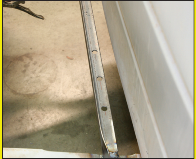
To facilitate welding, three holes were drilled in the new frame mount.
